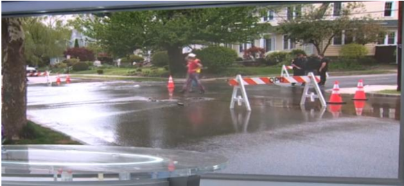
Water main break May 2, 2026 Courtesy News 12
